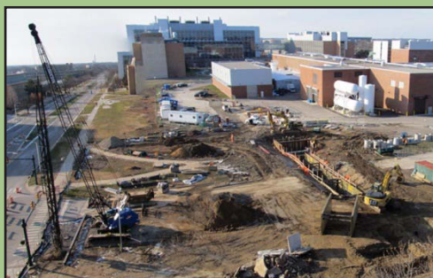
Work is ongoing to relocate steam tunnels and other utilities from under the footprint of future FRIB buildings. Other activities to prepare the site for the start of civil construction continue on schedule for completion in April 2012.
